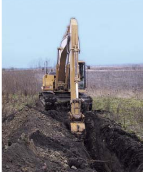
Crews removed 11 miles of agricultural drain tiles in the Rollins Savanna preserve.
